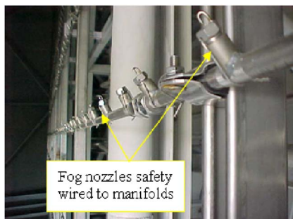
Fig. 2 Typical high pressure nozzles in an intake duct [4]
