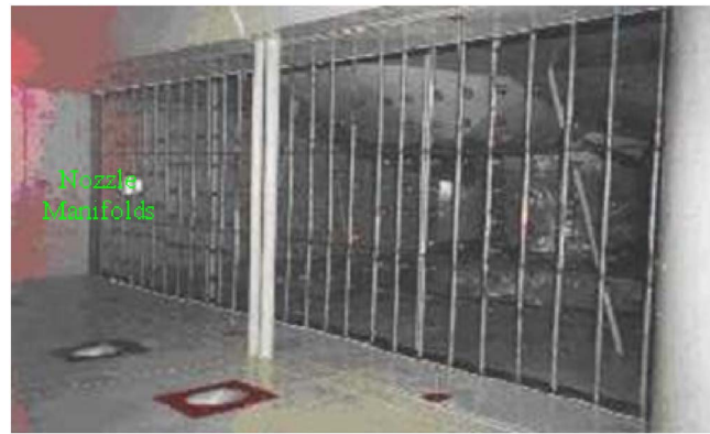
Fig. 14 Nozzle array mounted in the inlet duct of Alstom GT24 gas turbine—a view looking into the intake cone (courtesy Caldwell Energy & Environmental, Inc.)
